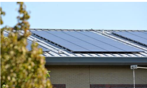
School solar PV installation
