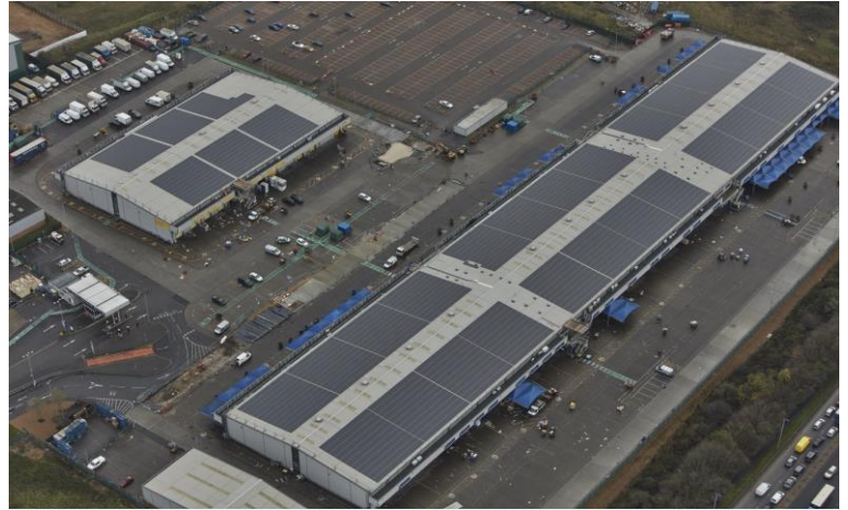
Solar PV installation at Western International Market
