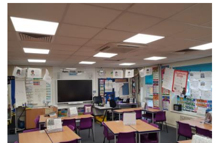
School LED installation
