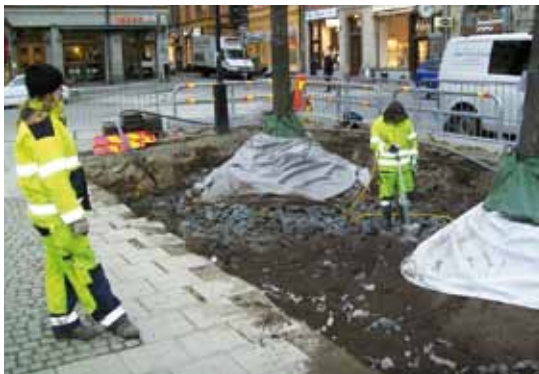
Root balls with new soil under protective cover and irrigation (notice the green watering bag around each tree). More soil is being flushed into the skeleton soil.
