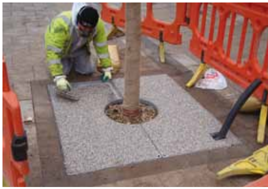
Grate with watering inlet and resin-bound infill and watering/aeration inlet on Ocean Road (see Case study 2, p31). Image: South Tyneside Council
