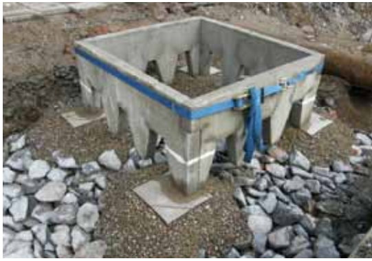
Positioning of concrete frame in continuous planting trench with large stones for skeleton soil along Hornsgatan, Stockholm (see Case study 25, p128).
