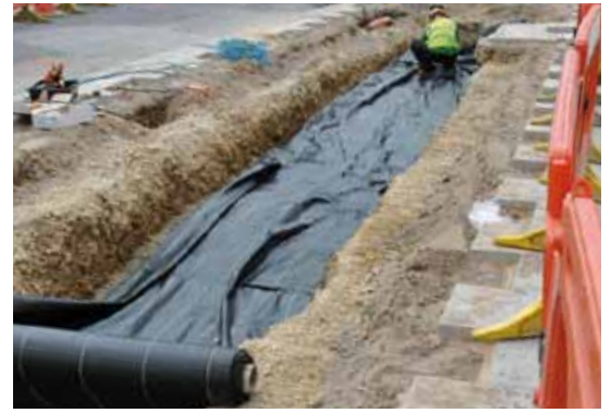
Root barrier lining.
