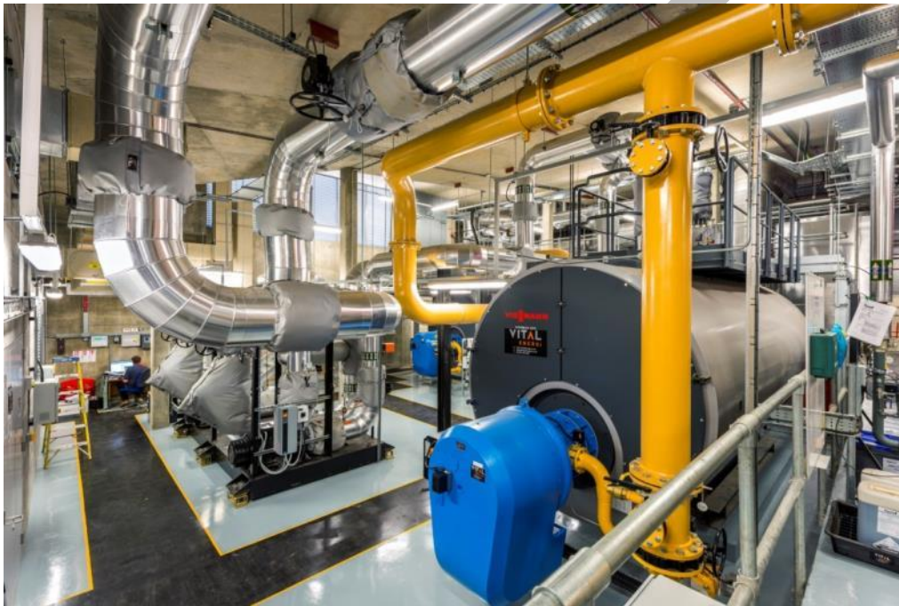
Figure 5.2 - Inside the King's Cross Energy Centre (reproduced courtesy of Vital Energi)
