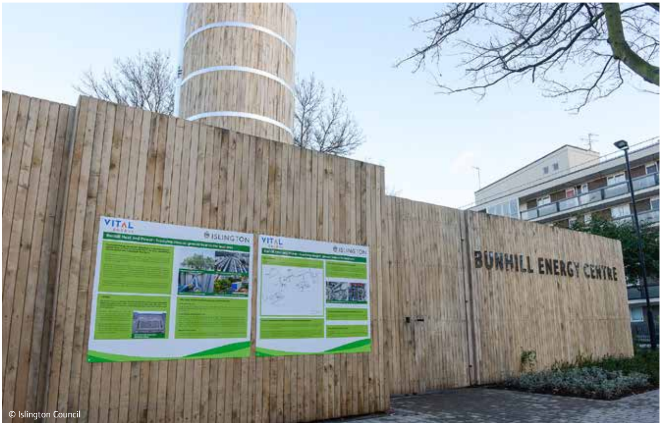
Figure 12. Thermal storage completed installation at Bunhill Energy Centre
