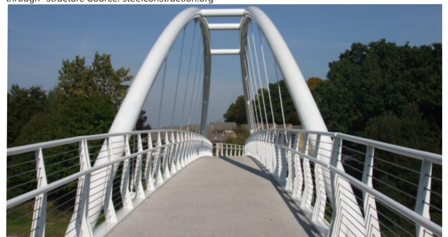
Figure 40: Mill Lane footbridge, a tied arch structure with the deck supported by high tensile hangers fixed to the bridge arches to suspend the deck. Source: NuSteel Structures Ltd
