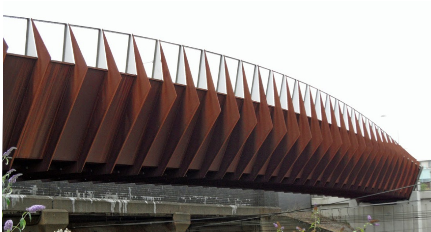
Figure 12: Shared use bridge in Queen Elizabeth Park over HS1 railway line; London, England. Source: Knight Architects
