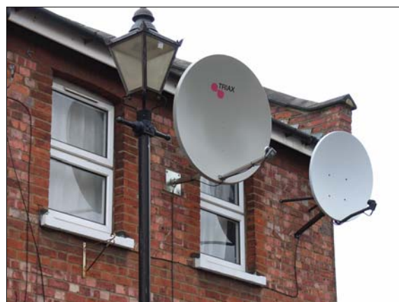
Proliferation of dish aerials on facades and other alterations harms the appearance of the street as a whole.
