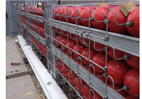
Hydrogen storage (compressed gas)
