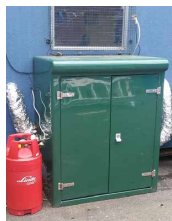
Remote site heat & power
