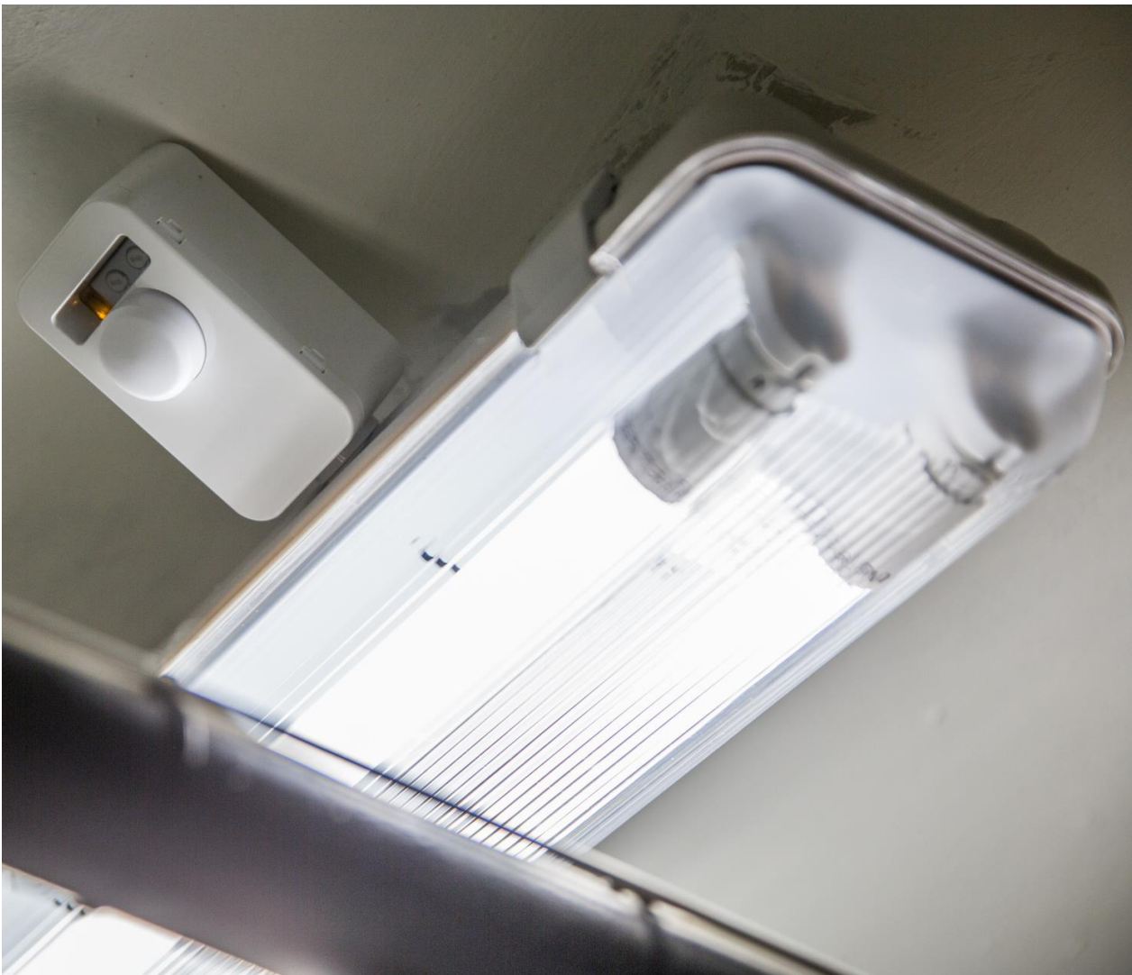
Highly efficient LED bulbs and motion sensors installed at Doddington and Rollo Community Association by Community Renewable Energy Wandsworth (CREW) in 2017, photo courtesy of CREW.
