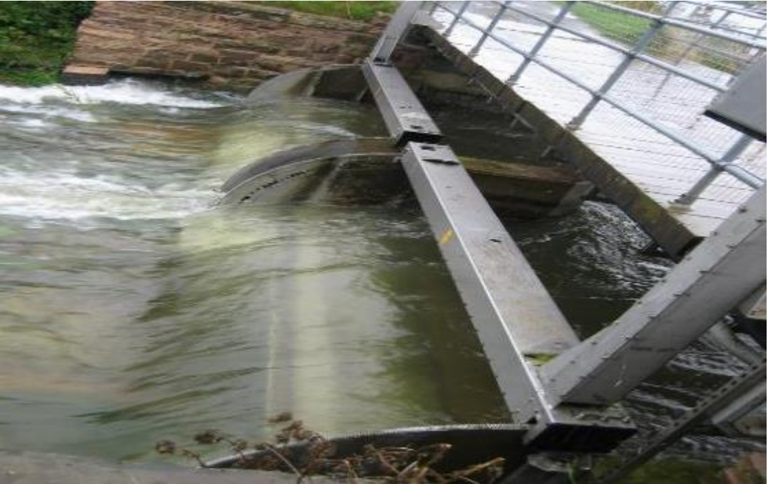
VI. Figure 6: Tilting weir gate – Purton Weir on Gloucester & Sharpness Canal
