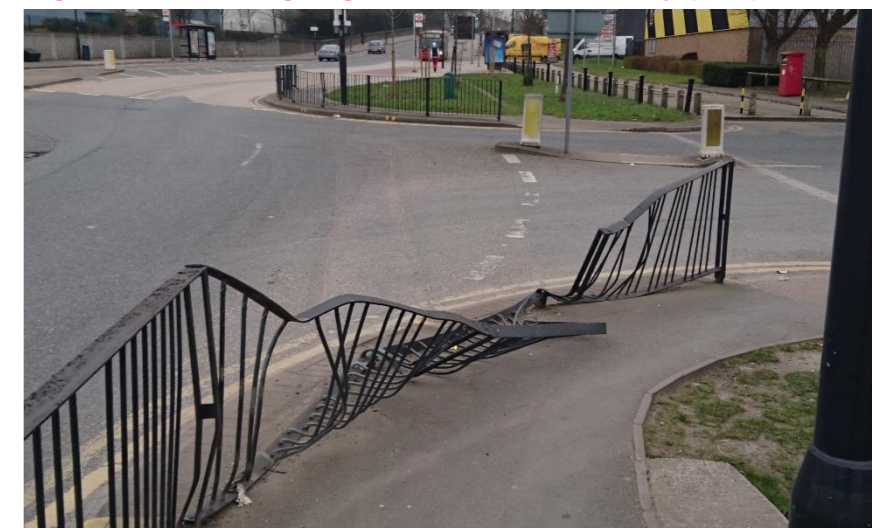
Figure 4-37: Damaged guard rail in the footway (C58)
