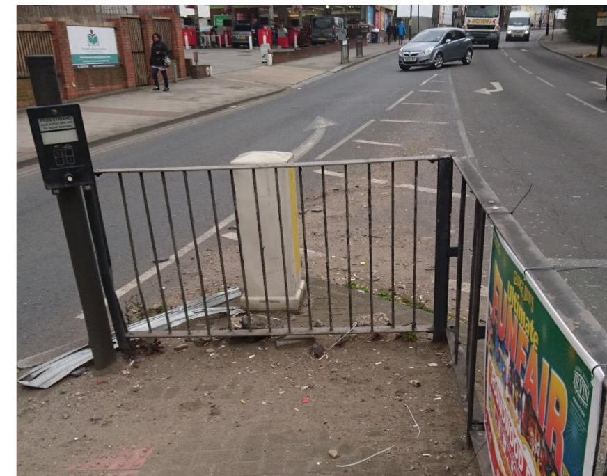
Figure 4-36: Build-up of grit and debris at crossing island (C7)
