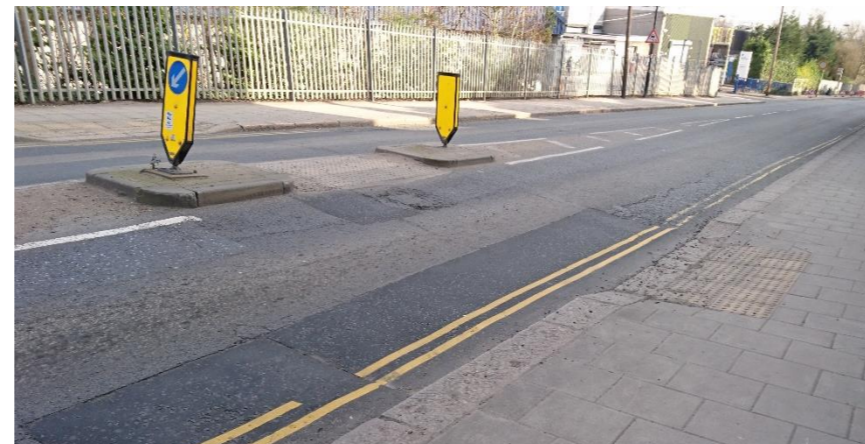
Figure 4-35: Carriageway damage at crossing (C22)
