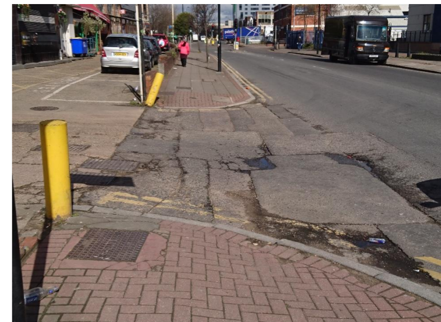
Figure 4-18: Poor surface quality at vehicle crossover (L23)
