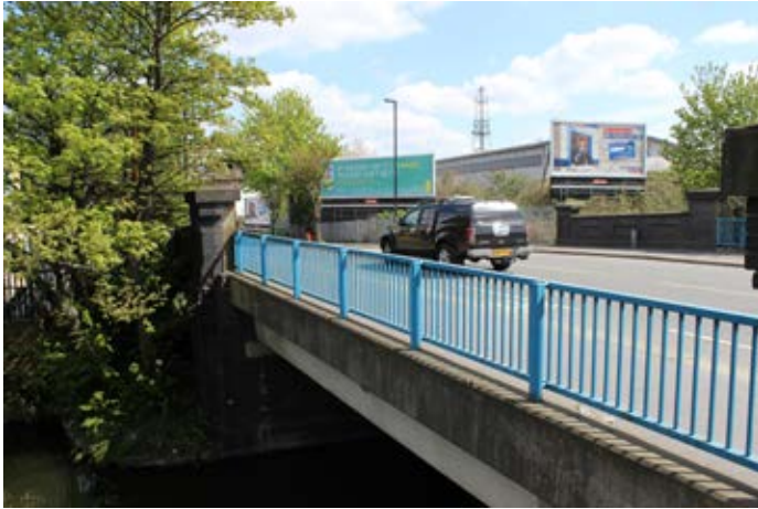
Figure 21: A view of Old Oak lane Overbridge from the south west (P6846010).
