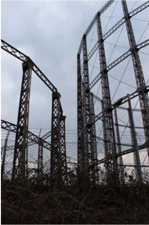
Figure 13: A detail of the gasholders. The larger and later Gasholder No 6, also known as 'the Colonel', is to the right (P6846005).
