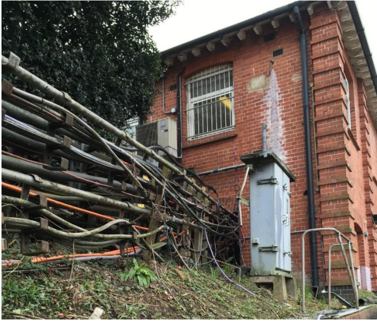
Figure 2.6: Cables running the length of the south side of the station
