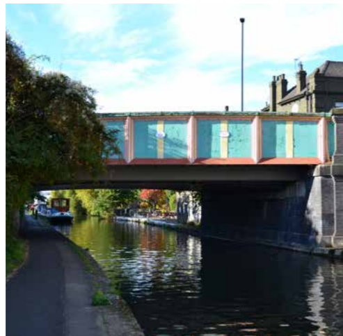
Acton Lane canal bridge, proposed as an 'other building of heritage interest'
