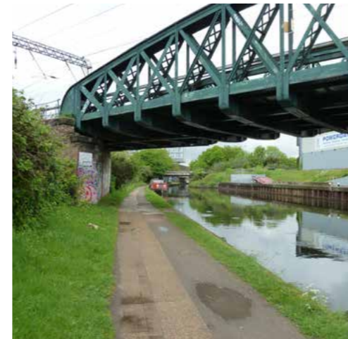
View looking west, the Kew Curve Grand Canal rail bridge crosses the canal near Powerday, recommended for local listing
