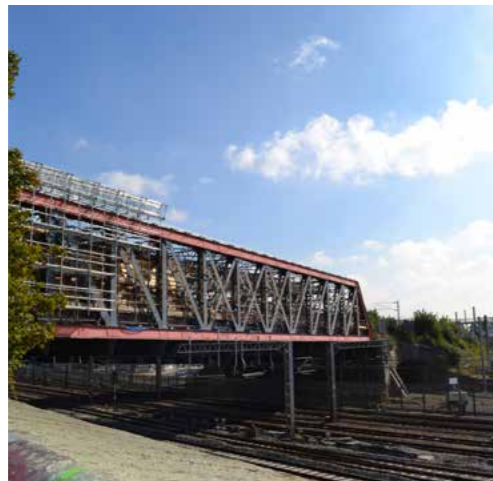
West London Line overbridge, a single-span skew bridge composed of braced steel trusses spans the Great Western main line, c. 1908, recommended for local listing
