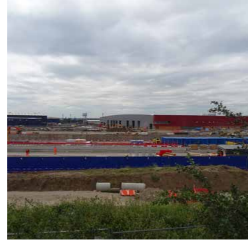
View looking south at the construction site of the new Crossrail depot for the Bombardier trains, which can be seen in the background
