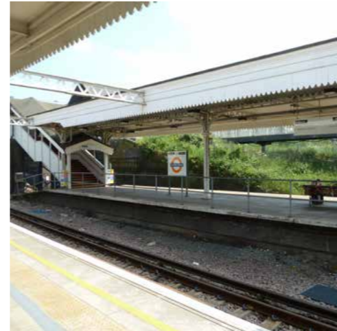
Willesden Junction Bakerloo and Euston-Watford low-level platforms still retain their original wooden canopies
