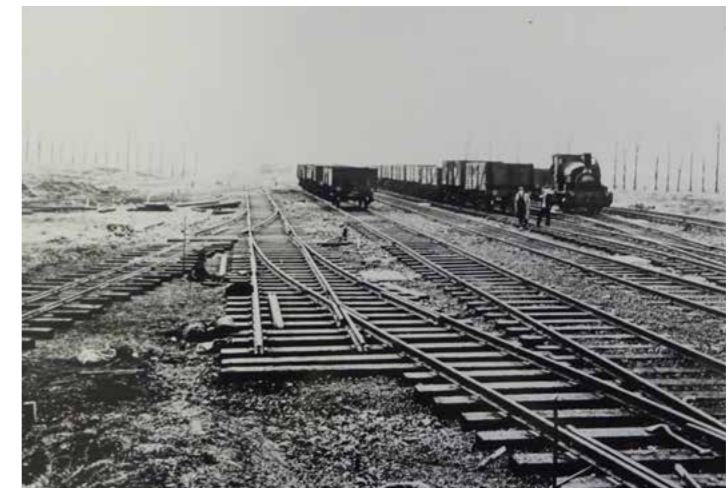
Railway sidings under construction at Guinness Brewery, 1934. Reproduced with permission of the Ealing Local History Centre
