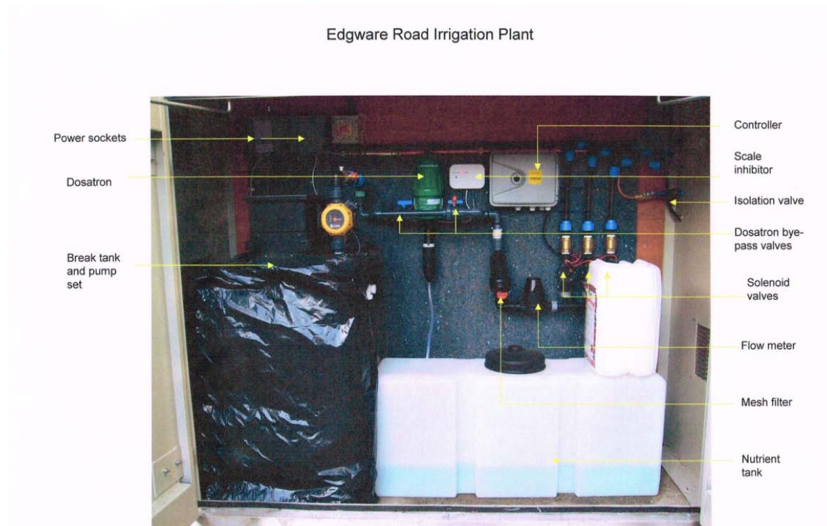
Figure 11: Edgware Road Green Wall irrigation plant
