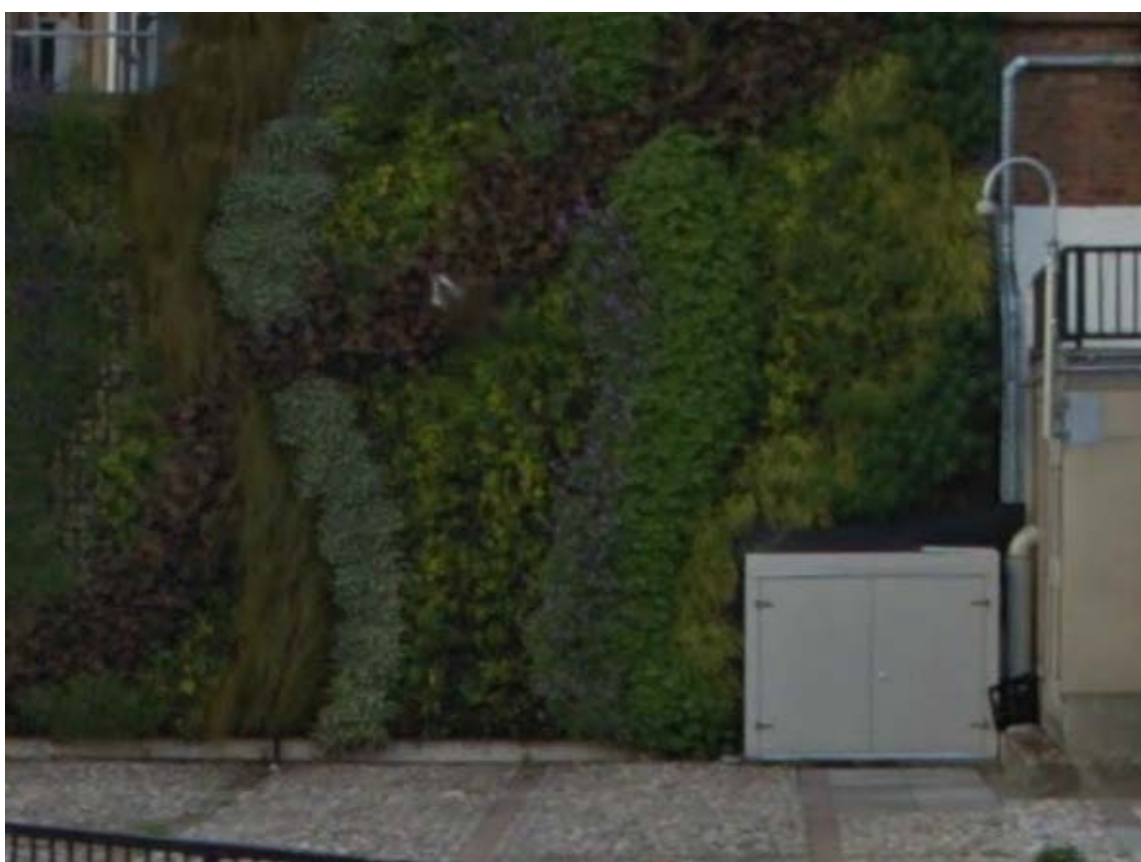
Figure 10: The pump cabinet
