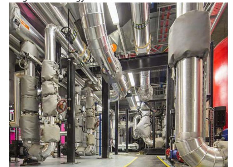
King's Cross Energy Centre
