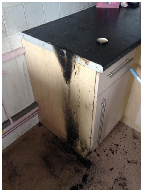
Damage to flat following sprinkler activation at Parkside Court (photo provided by CHP)
