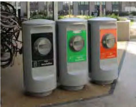
Figure 9.5: pneumatic waste collection system at Wembley
