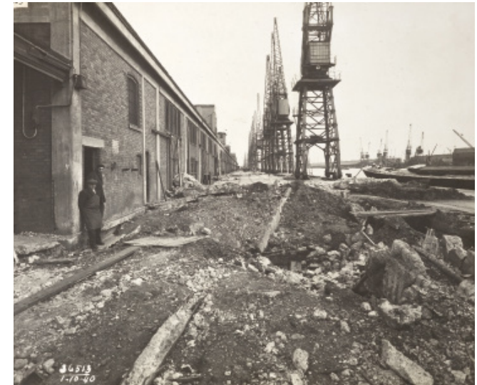
AIR RAID DAMAGE AT ROYAL ALBERT DOCKS, 1940 © PLA collection/ Museum of London
