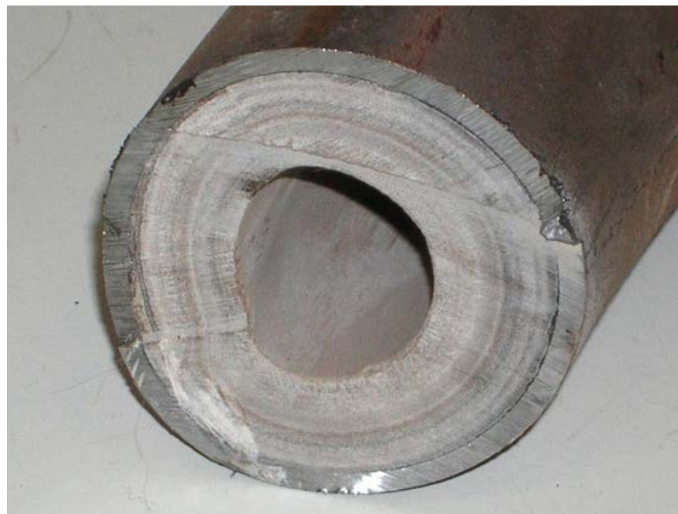
AN INDUSTRIAL PIPE THAT CARRIES WATER
