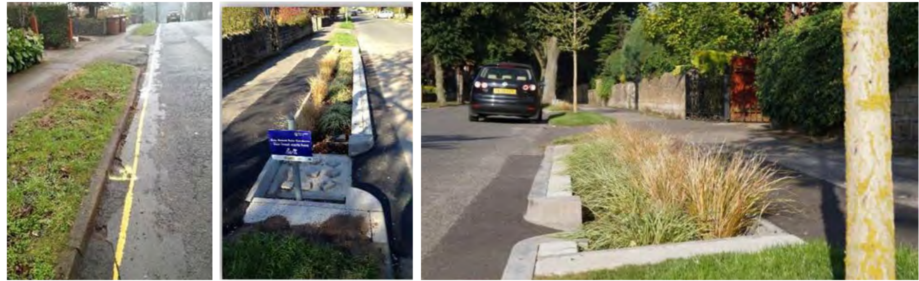
Figure 5.13 Greening streets, retrofit rain gardens at SuDS Project in Ribblesdale Road, Sherwood (before and after)
