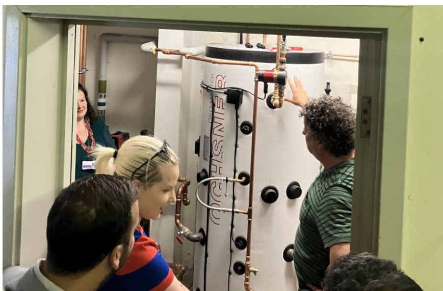
Figure 3: Members of the Committee and Stokey Energy inspect the air source heat pump system in the Clubhouse
