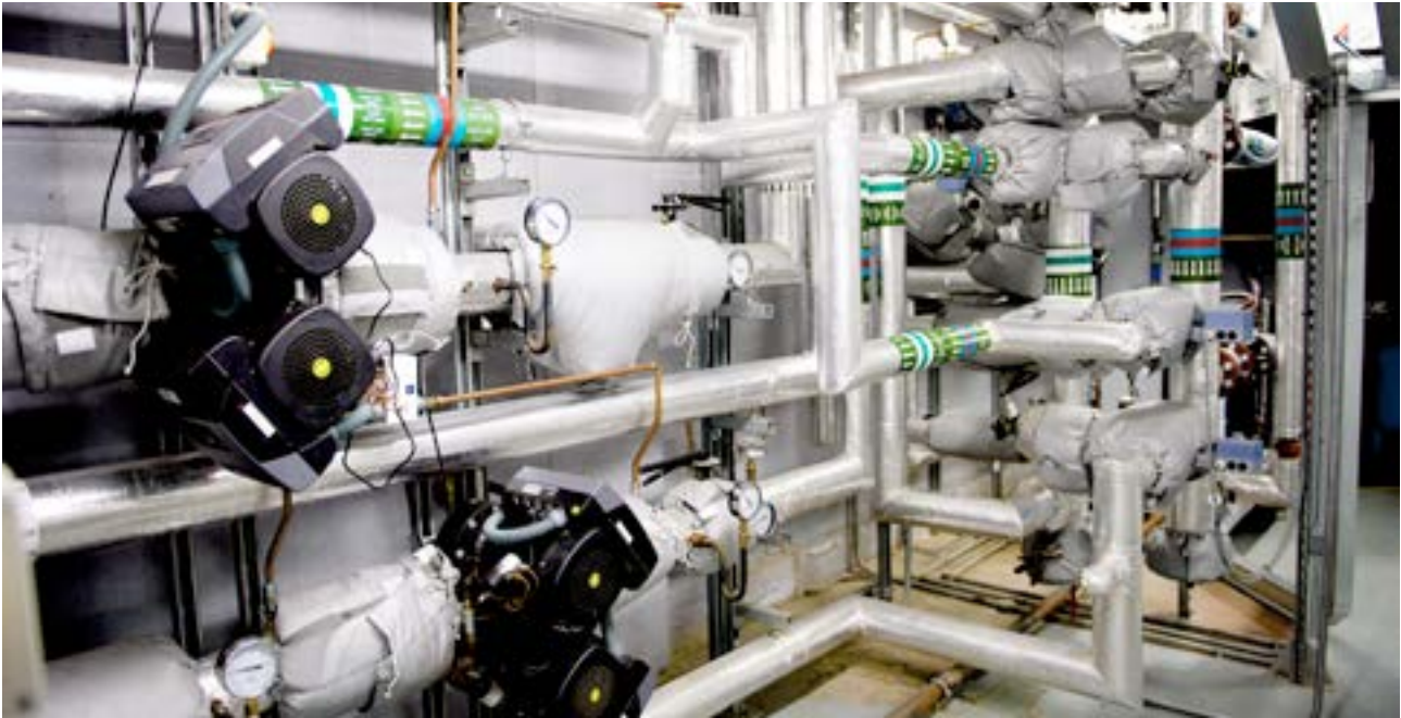
Bunhill Energy Centre, an Innovate UK-funded smart cities demonstrator project
