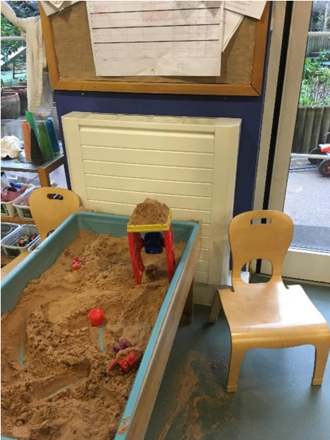
Radiators cabinets in main classroom
