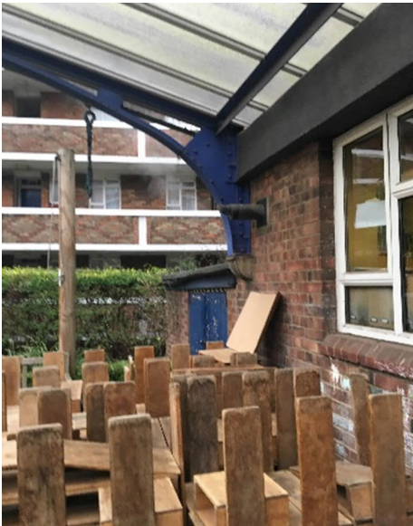
Boilers vent their exhausts from the wall into the main playground
