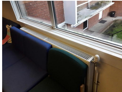
Radiators valves that assist in controlling temperature
