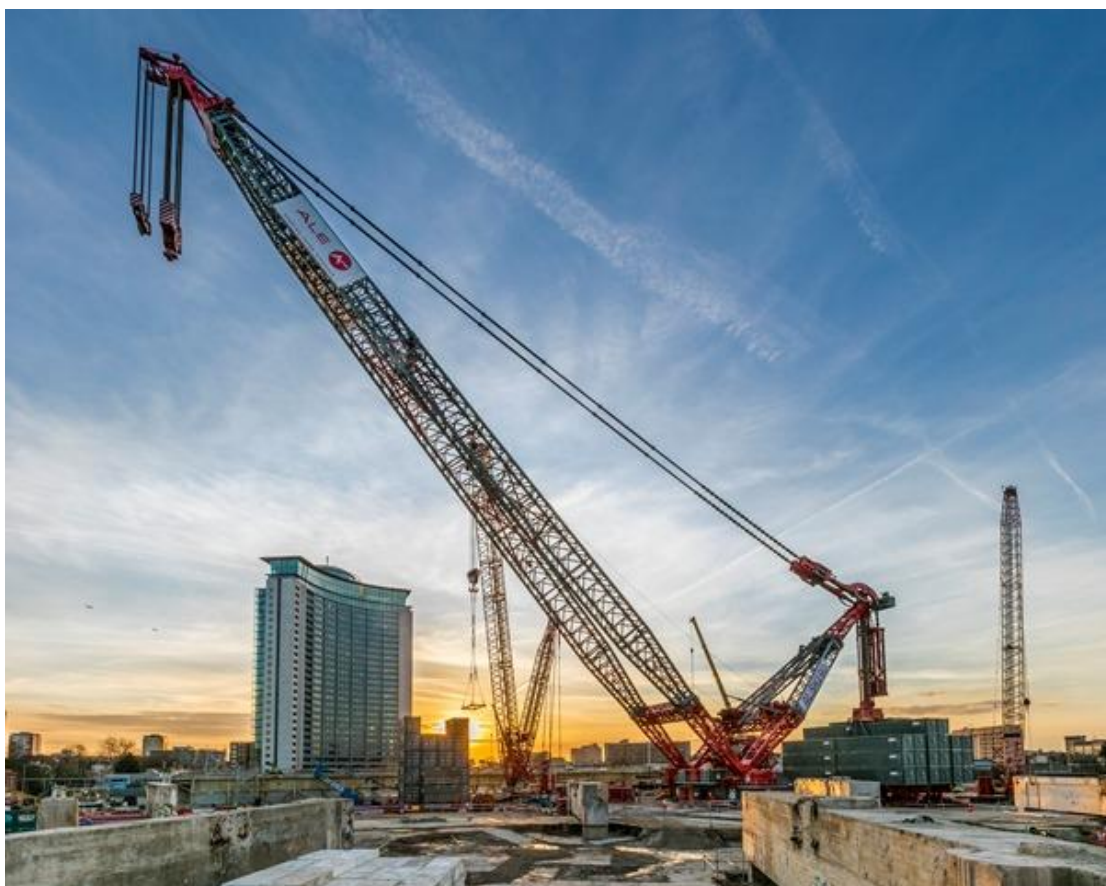
Fig. 1: Image of the Heavy Lifting Crane used to remove the 61 ‘portal’ beams
