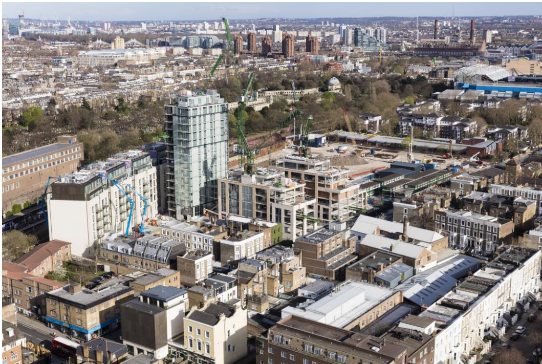
Fig. 5: View of construction progress on the Lillie Square development (looking south from Earls Court masterplan site)
