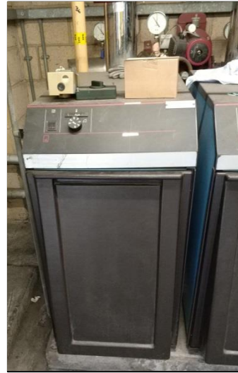
Aging gas fired boiler
