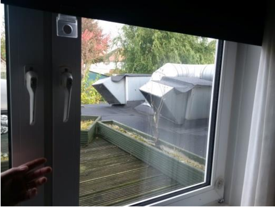
Kitchen extract from caretaker flat window
