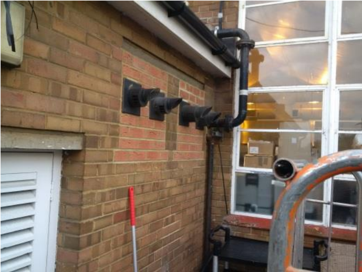
Boiler flues from nursery plant room into commercial kitchen delivery area
