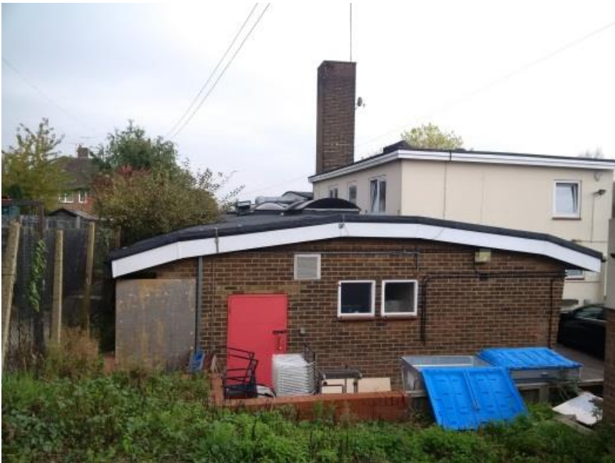
Kitchen building, air extract and flue tower
