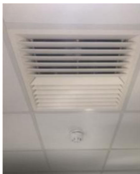
Modern air conditioned building
