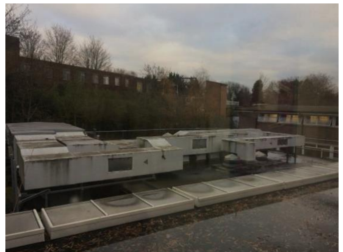
Extensive ventilation equipment on the roof of the kitchen
