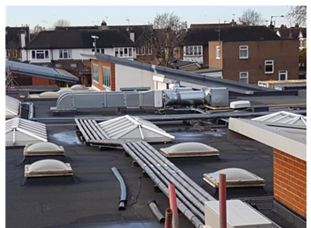
Air Handling Units
