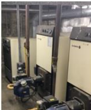
Ageing boilers in plant room
