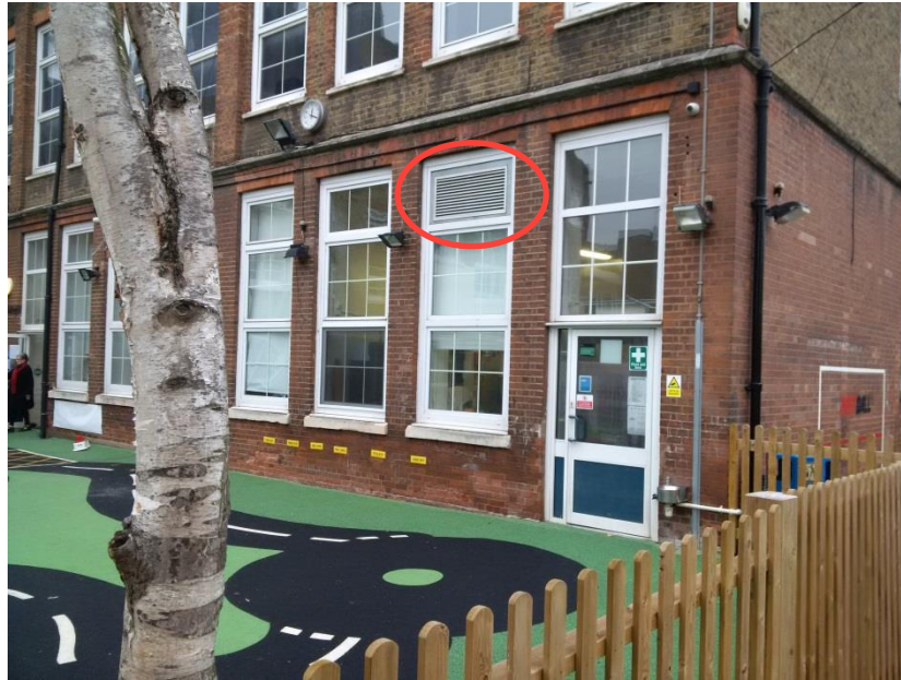
School kitchen extract discharges into school playground
