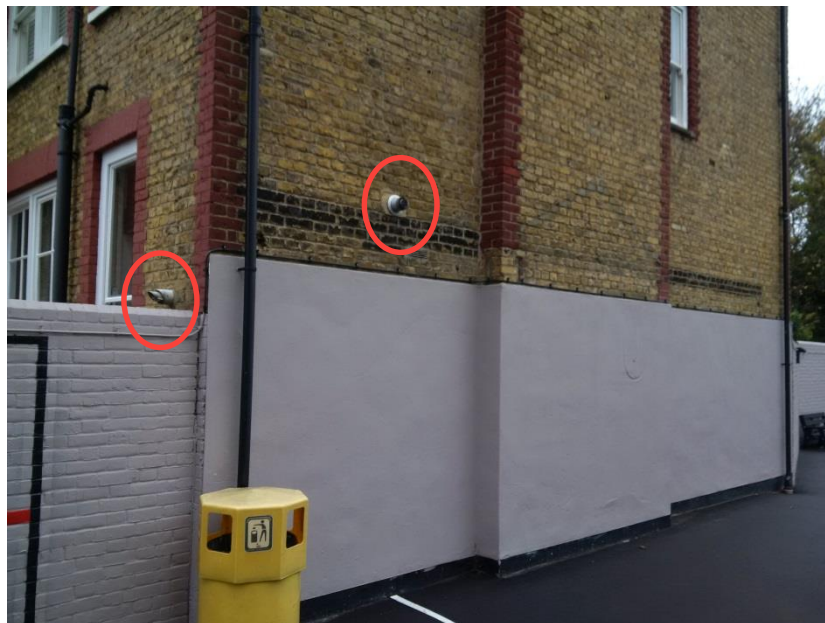
Two gas boiler flues from ex-caretaker house discharging into school playground
