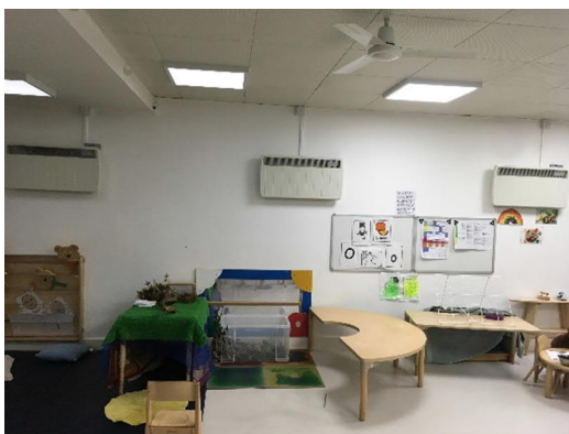
Air Conditioning Units in upstairs classroom
