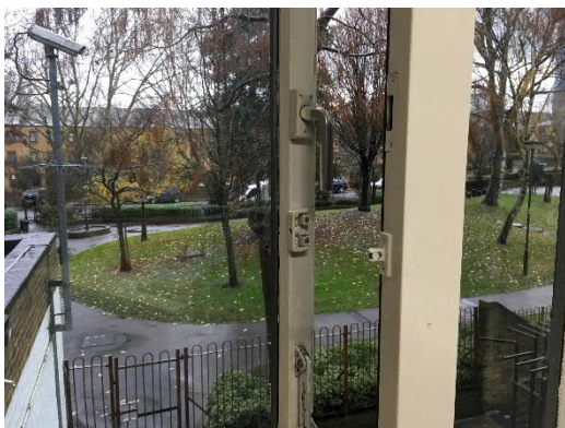
Opening of windows for natural ventilation
