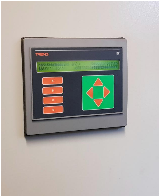
Boiler trends board corrupted
