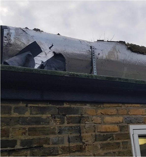
Insulation lagging for kitchen extract coming away
