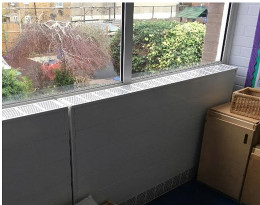
Older heating units on upper floor; issues with control units prevent these from being switched off in summer
