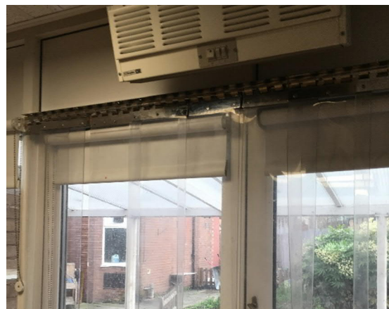
Heat curtains on main doors used to help prevent heat loss when open. Older heating units visible above door.
