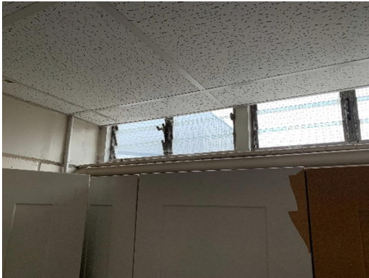
Older single pane slatted windows; key area of heat loss and in-efficiency
