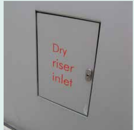
Dry riser inlet considered in relation to facade ✅
