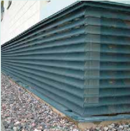
Inappropriate venting to undercroft parking ❌
