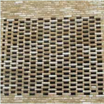
Appropriate venting to facade ✅
