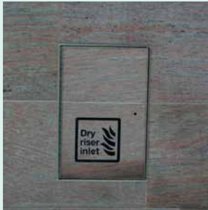
Dry riser inlet considered in relation to facade ✅
