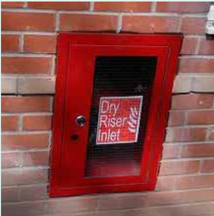
Dry riser inlet not considered in relation to facade ❌
