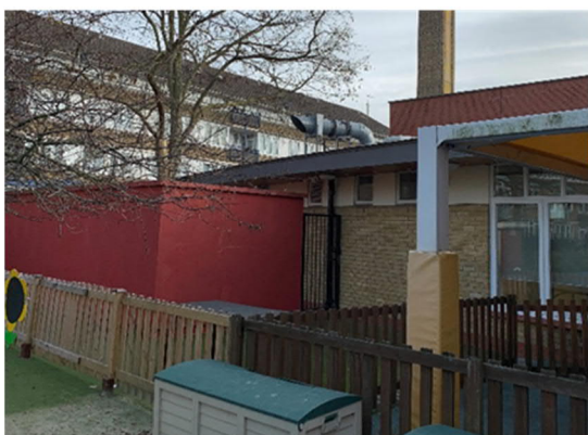
Main Playground – Heat extraction from rood in proximity of outdoor play space
