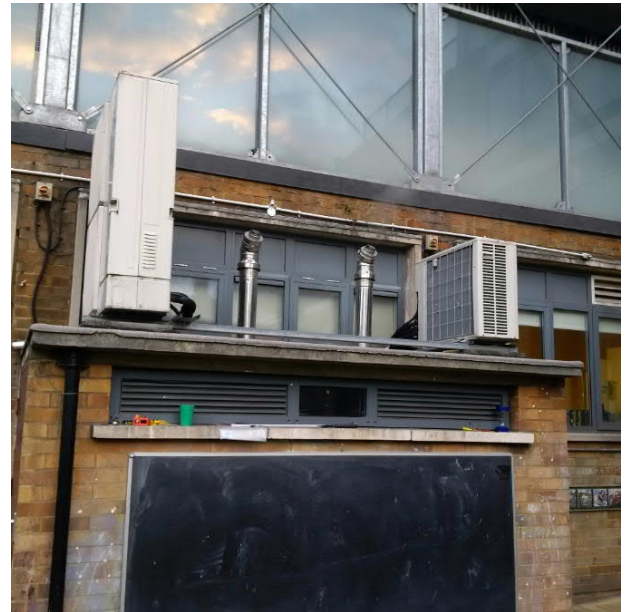
Two gas boiler flues exhausting into nursery courtyard garden
