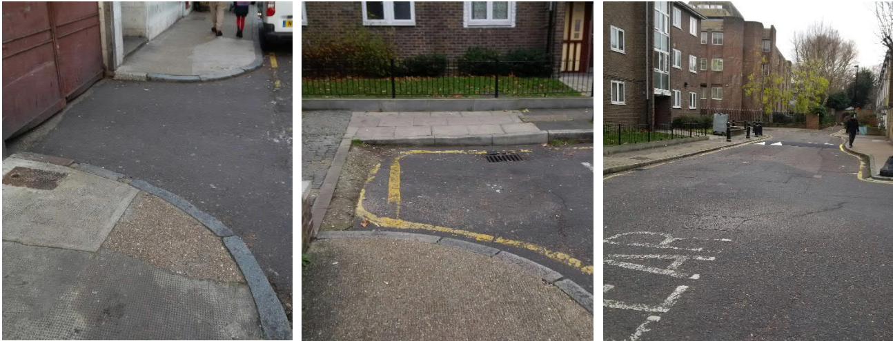
Missing drop kerbs and cluttered footway Beaumont Grove
