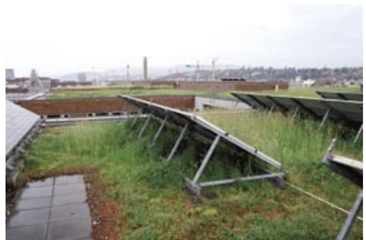
Photovoltaics and Green Roofs, Switzerland. Photo: Livingroofs.org
