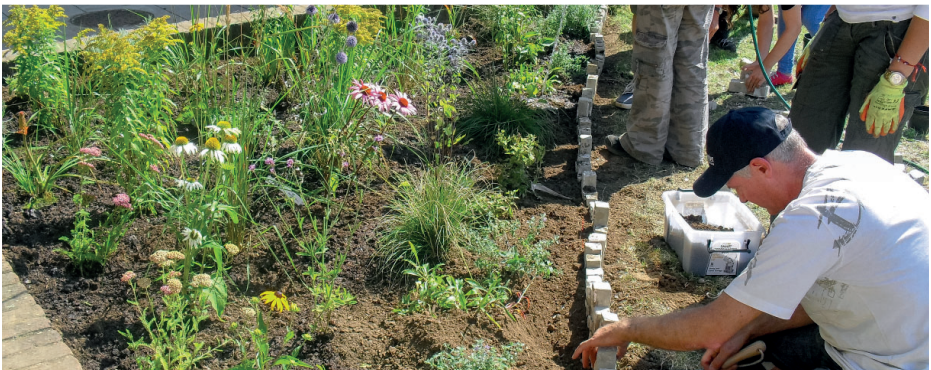
It is important to check for underground services before digging.
